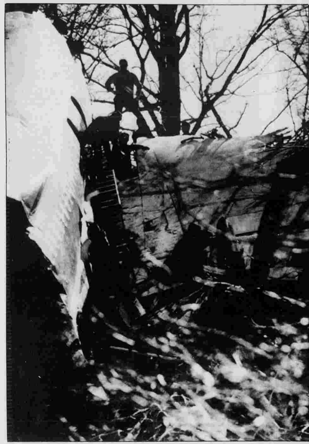
Workers use chainsaws to hack through the wings of the Avianca jetliner which crashed last week on Long Island. Crews began removing the wreckage Thursday.
